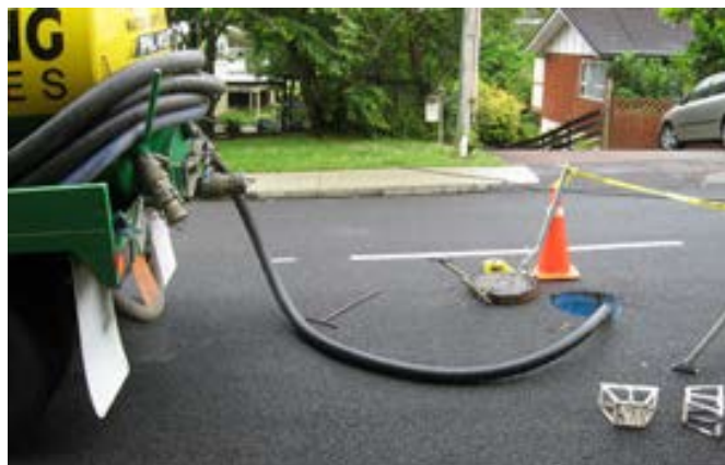
Figure 2: Sediment is removed from the sump with a vactor hose. Confined space entry is not required for this step.
